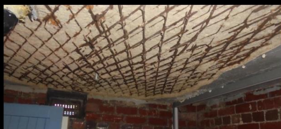
Large area of concrete soffit spalled whilst hammer testing. Spalling caused by erosion of steel mesh reinforcement.
