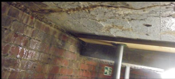
Cracking to below concrete soffit with water droplets appearing on surface, evidence of continuous water ingress.
