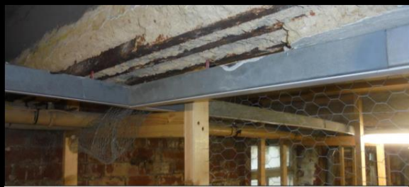
Large area of concrete spalled from structural beams showing eroded steel reinforcements.
