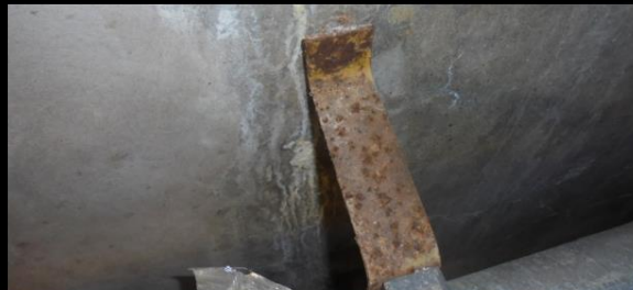
Services have been fixed into tanked pool wall allowing water to penetrate through in places
