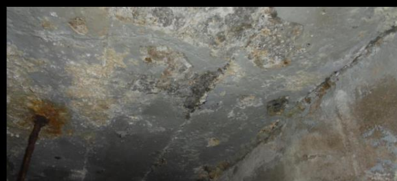
Hammer test revealed large areas of the concrete soffit which are hollow with evidence of continuous water ingress from above.
