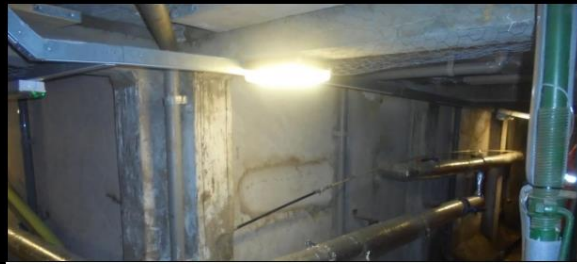
Pool walls and columns have been previously tanked but survey has revealed the system has failed with large sections sounding hollow and there is evidence that water is penetrating through.
