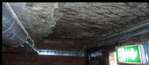
Further example of spalled concrete caused by erosion of mesh reinforcement.
