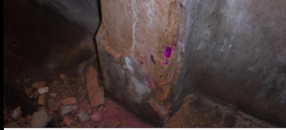
Another example of spalled render to the columns with signs of water penetrating through.
