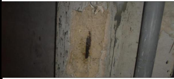
Structural column reinforcement has become eroded causing concrete material to spall along with surface render
