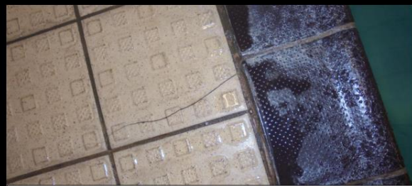
Close up of hairline cracking to walkway tiles which we noted in various areas around pool.
