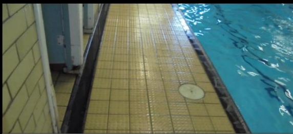
Pool walkway is not water tight allowing ingress to concrete floor slabs and supporting columns and beams below.
