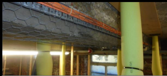
Wire mesh used as a safety measure preventing spalled material falling from concrete beams.
