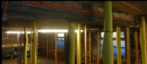
Previous repairs on beams have failed due to the continuous rusting and expanding of steel reinforcements.
