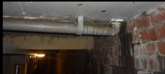
Further image of cracking to walkway concrete soffit.
