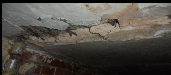
Previous repair attempted using sand cement repair which has failed revealing rusted steel reinforcements
